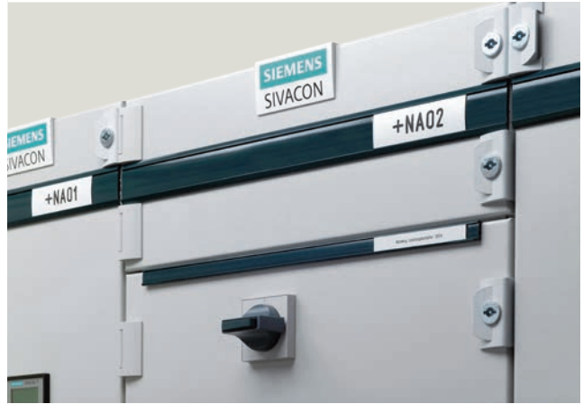
Standardised labeling system for cubicles and feeders
