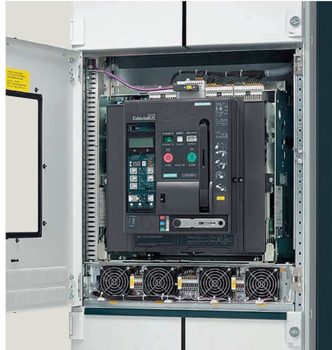
Cooling system with fans underneath the 3WL circuit breaker
